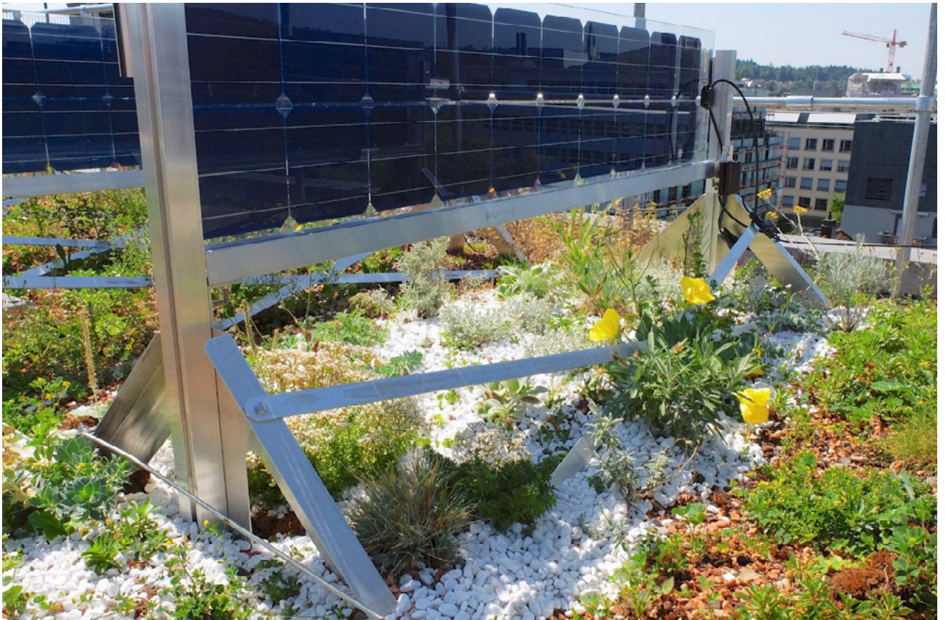
Figure 18: Installation test de la ZHAW, source: Solarspar
